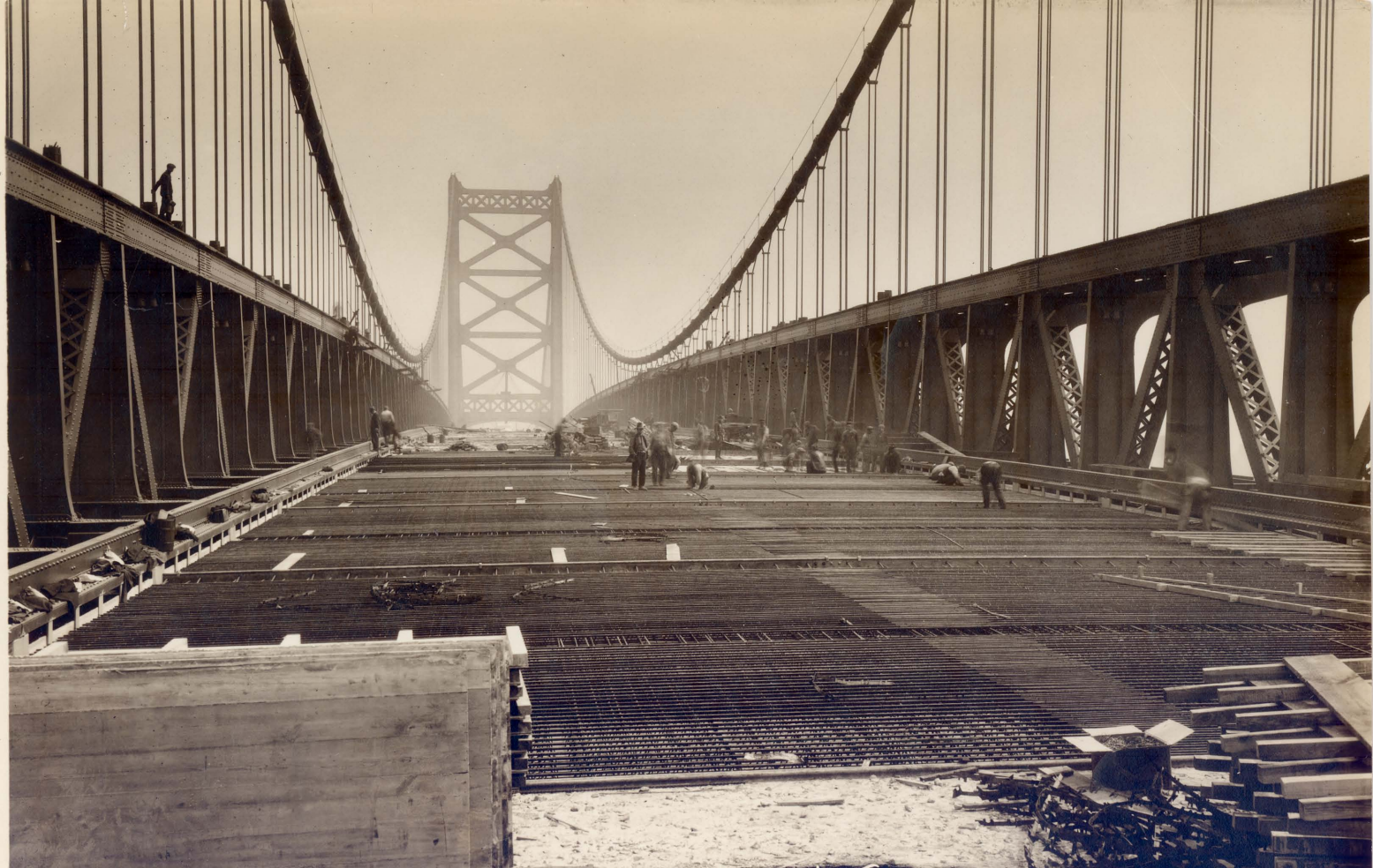
2421 Bridge Roadway Reinforcing on Main Span East of Phila. Tower - Looking East 10-8-25
